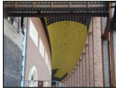
Barrel vault soffit that curves around the colonnade perimeter of the stadium was sheathed with fiberglass matte faced gypsum sheathing.
