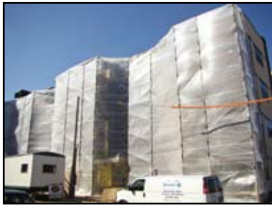
Process of stuccoing is complicated by cold weather. Stucco 1's capable crew provided plastic sheeting and heat to scaffolding of Phase II of the Van Cleve project.
