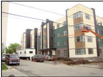
Scaffolding and tenting comes down to reveal the nice finishing work by Stucco 1's plasterers.
