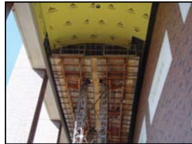
Staging was supported by hex lifts that brought the Mulcahy crew right up to the work area fifty feet above the colonnade.
