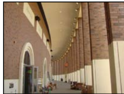
A shot of the finished soffit completed in a direct application of Parex mesh reinforced base coat and acrylic finish.
